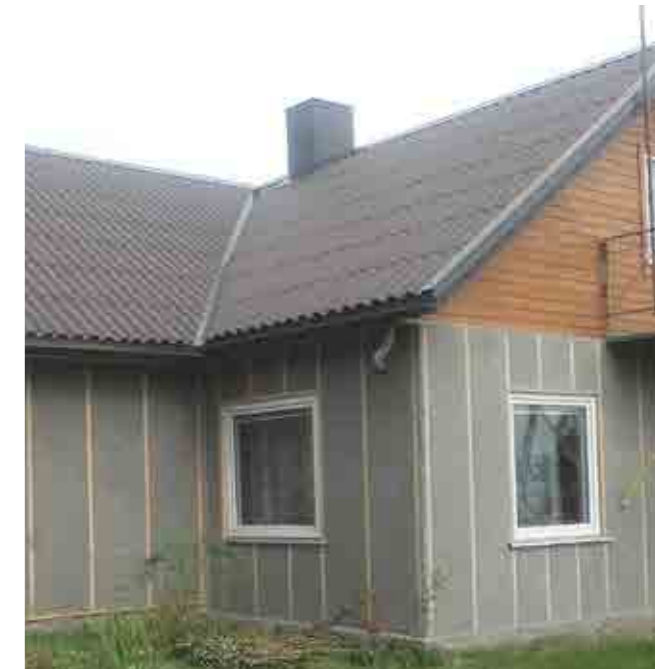
While replacing the roof, we have renovated the whole house as well
